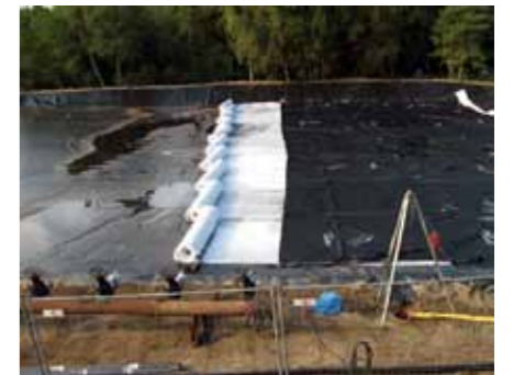
Geocomposite drain placed over geomembrane liner prior to placement of Geotube ® containers
