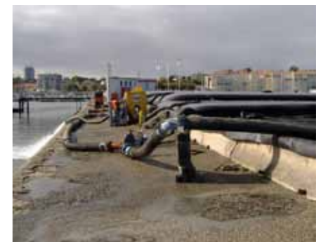
Returning effluent water to marina basin
