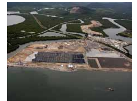
Geotube ® dewatering of contaminated sediments in the first cell while preparing the second cell
