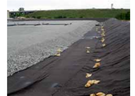
Geomembrane lined drainage platform for the dewatering platform
