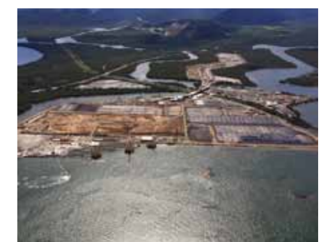
Surcharging the first Geotube ® dewatering cell while operating the second Geotube ® cell
