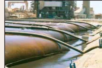
Geotube® containers at fossil fuel power plant being used to dewater fly ash.
