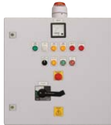
30kW Pump Control Panel
